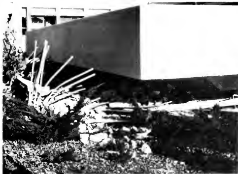
Photo 36. Psychiatric Unit, with first story roof now on the ground. Dowels (reinforcing steel from footing) show that building moved laterally during failure.
